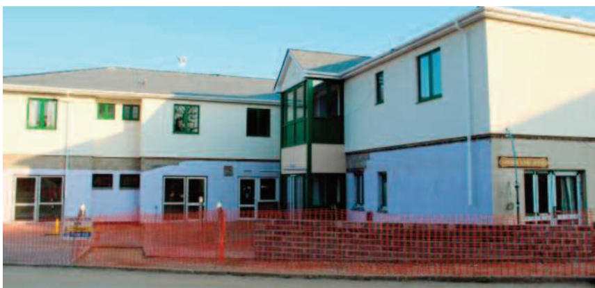
Forder Lane House undergoing renovation (March 2012): South Devon Rural Housing Association’s Retirement Home
